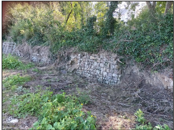
The retaining wall at Marhamchurch Wharf at the top of the incline which has recently been revealed following some clearance work by the landowner.
