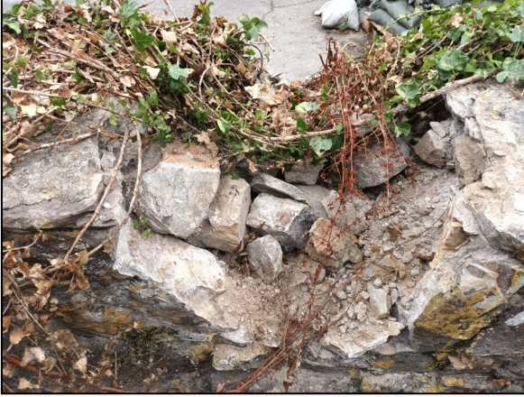
The wall in front of the entrance to Helebridge House which appears to have been damaged during an attempted demolition
