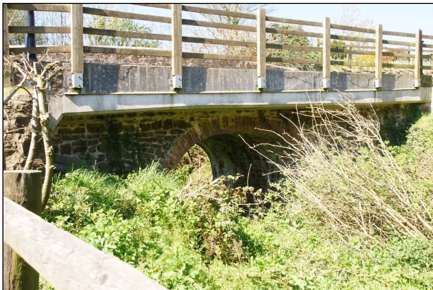
Burmsdon Farm Bridge which is on the section of canal mentioned above
